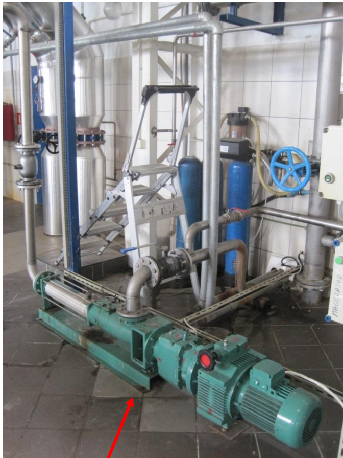
Pump dosing waste to AD
